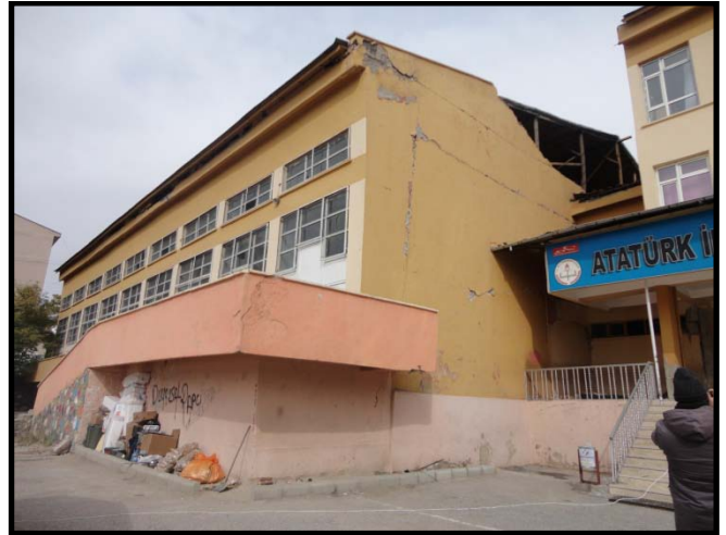
Fotoğraf/Picture 67 – Minimum Hasarlı Spor Salonu - Ercis / A Sport Hall with Minor Damage - Ercis
