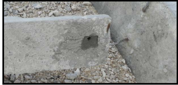
Fotoğraf/Picture 80- Grout Hasarı / Insufficient Bond Characteristics and the Resulting Pull-Out Failure
