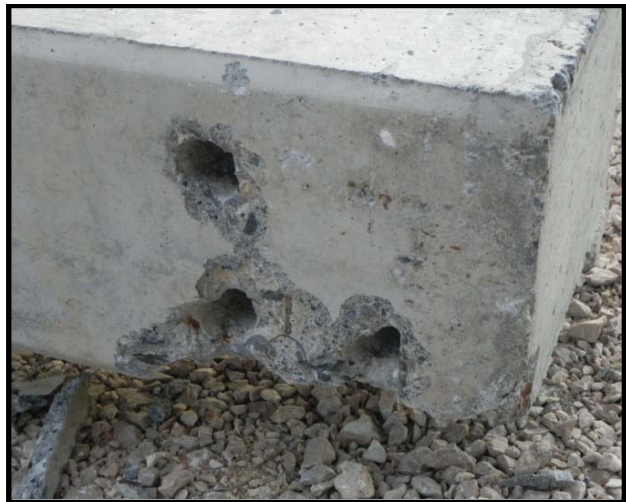
Fotoğraf/Picture 84- Unutulan 4. Delik / The Missing 4 th Hole for Beam-Column Connection at the Beam End
