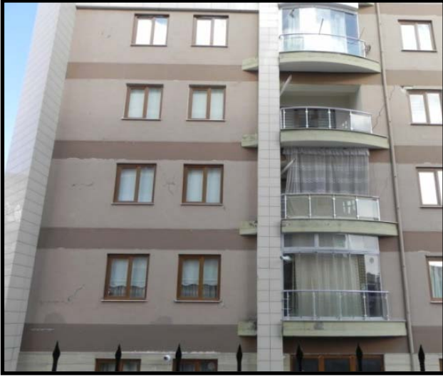
Fotoğraf/Picture 73 – Ard-germeli Yapıda Duvar Hasarları / Damage on Facade Walls of the Frame Building with Post-tensioned Connections
