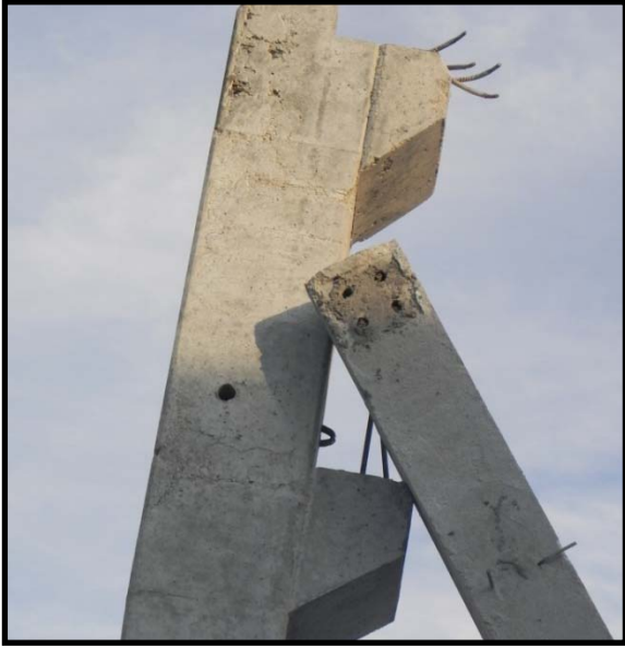
Fotoğraf/Picture 79- Mesnetlerde Aderans Göçmesi / Bond Failure at the Beam to Column Connections
