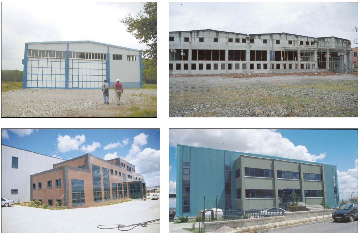
Figure 3 – Typical Single- and Multi-Storey Warehouses after Kocaeli Earthquake [5]
