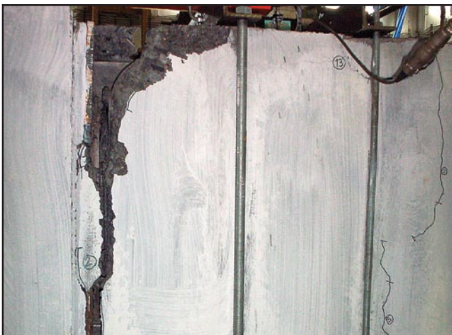
Fig. 17. Damage in bolted specimen at 4% drift level.
