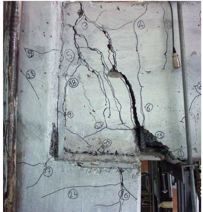
Fig. 14. Damage in composite connection specimen at 3.5% drift level.
