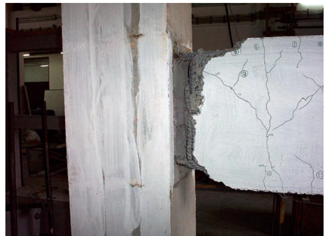
Fig. 11. Damage in specimen cast-in-place in column connection at 4% drift level.
